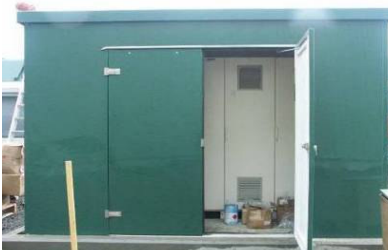
MCC located in small "porta-cabin" building
